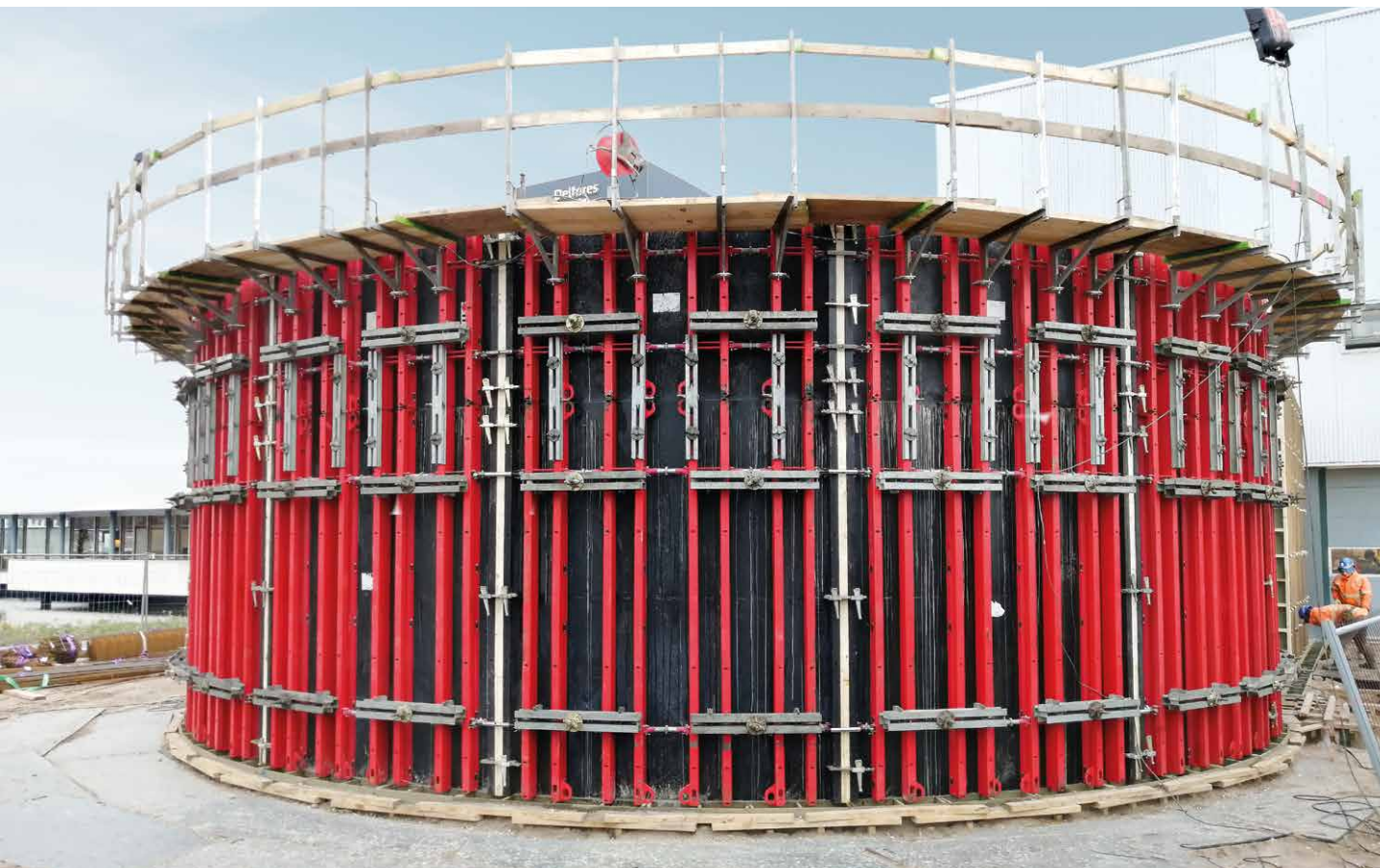
Perfectly round and with a constant radius from the ground to the ceiling: the research centrifuge required perfect formwork.
