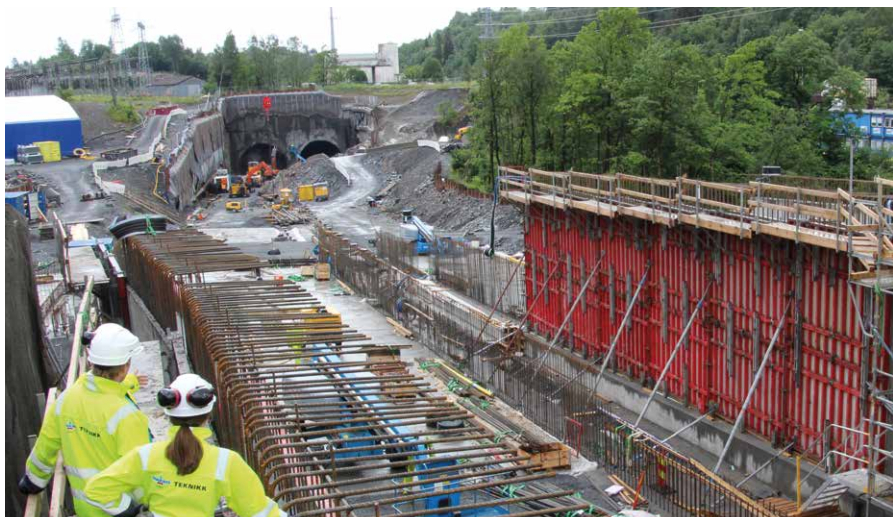
The simple handling of the AluFix formwork paid off in the confined space in the tunnel (left). In front of the tunnel entrances (top), Mammut 350 ensured rapid construction progress.
