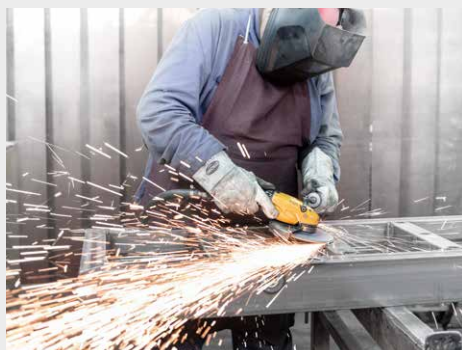
Additional works in case of damage All mechanical repairs to panel frames
